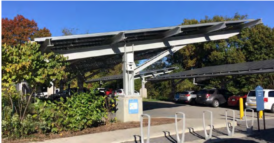
Figure 11 – Example, Carport Mounted PV System
