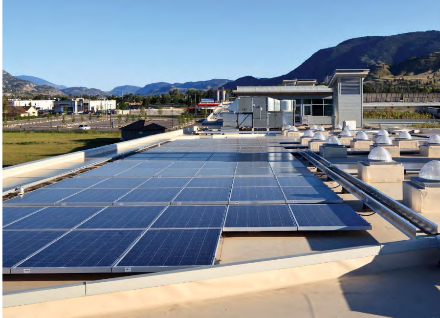
Figure 8 – Example, Roof Mounted PV System
