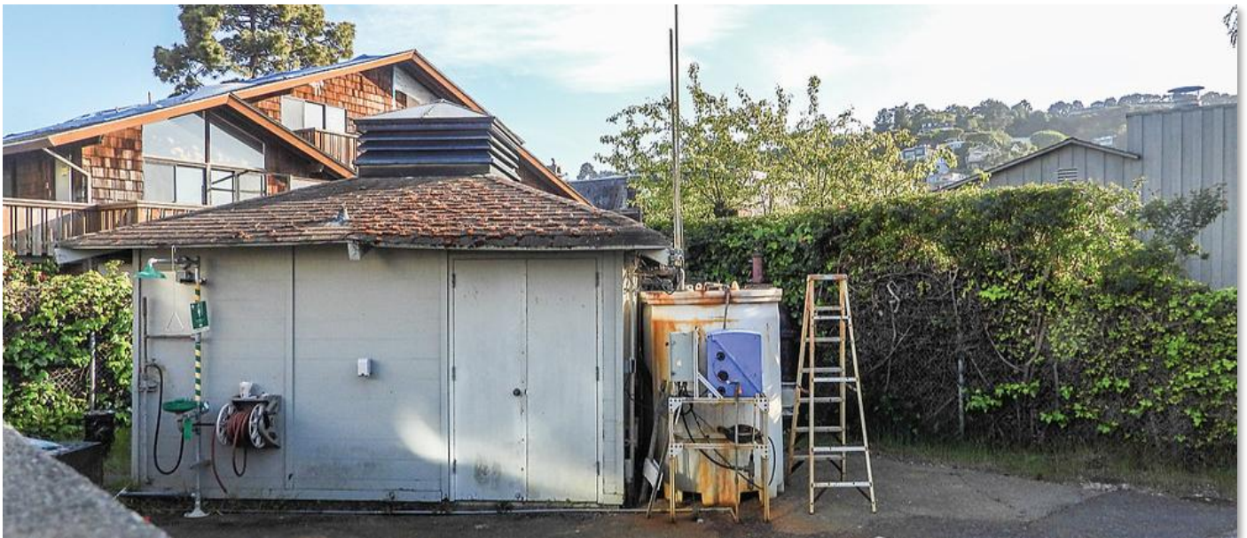
Cove Road Pump Station | One of 24 SD5 Collection System Pump Stations
