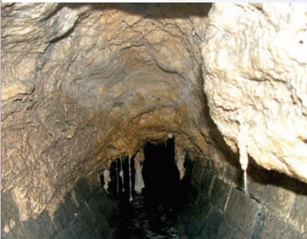
Disposing of F ats, O ils, and G rease down the drain can quickly lead to clogs like this! Do your part to keep FOG out of the sewer system.
